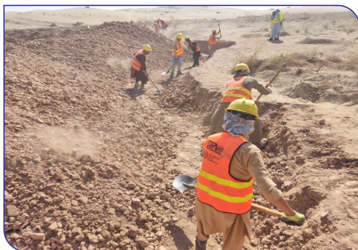
Figure 1: Excavation of selected material from quarry using labour for road levelling work on Shortepa district road rehabilitation project, Rabat village in Shortepa.
