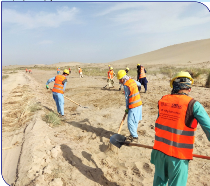
Figure 1: Road formation activity at a section of the Shortepa District Road Rehabilitation, (Ch. 1+100-2+100), in Balkh district.
