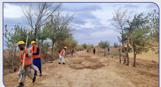
Figure 2: Preparation of the subgrade on the Bazar Jangal Ariq to Jangal Ariq Watani road, Ch 1+360 - 2+520, Jawzjan district
